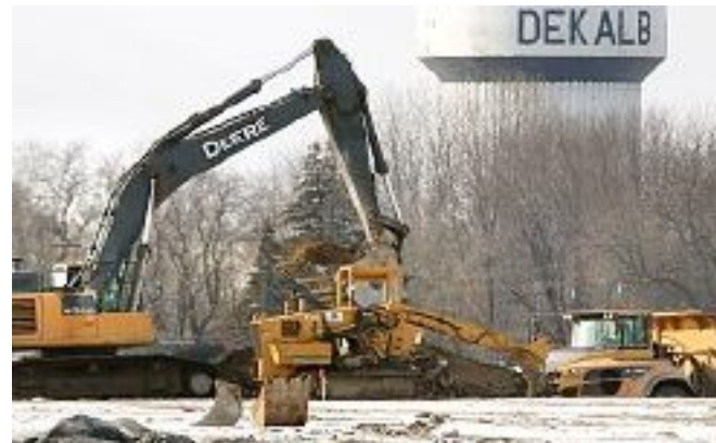
An excavator moves dirt Mark Busch Friday at the ChicagoWest Business Center in DeKalb.
